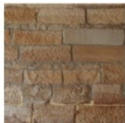
1 Sandstone Blocks EXISTING SANDSTONE BLOCKS ON SITE TO BE RETAINED AND CLEANED
